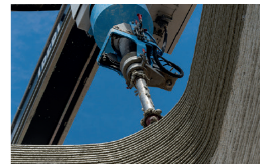
3D concrete printing offers design freedom and construction efficiency. Heidelberg Materials supplied 333 tonnes of 3D concrete printing material for the largest 3D printed building to date in Europe. Read more on p57.
