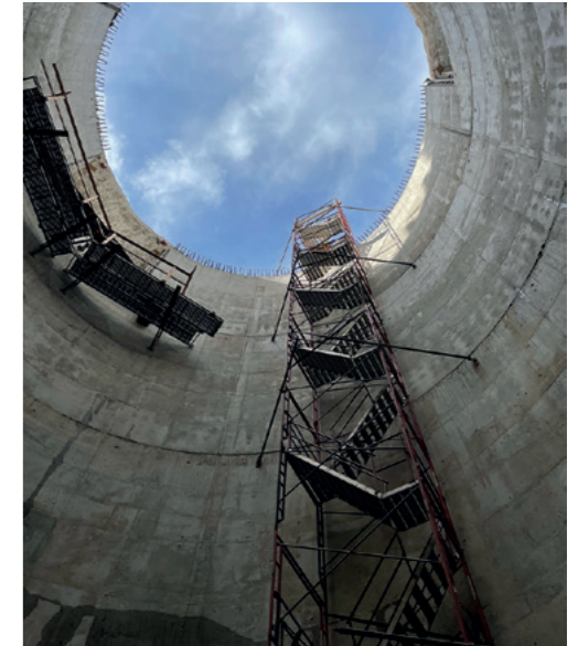
In the USA, the NRMCA 2024 Concrete Innovations Awards went to 10 projects that used innovative product to lower the project embodied carbon. CO 2 reduction of 21% was achieved at this stormwater storage facility. Read more on p64.
